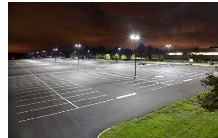
Industrial Lighting Control
